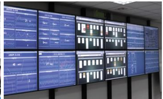
Green Light control room is awake all day and all year round for continuous operation
